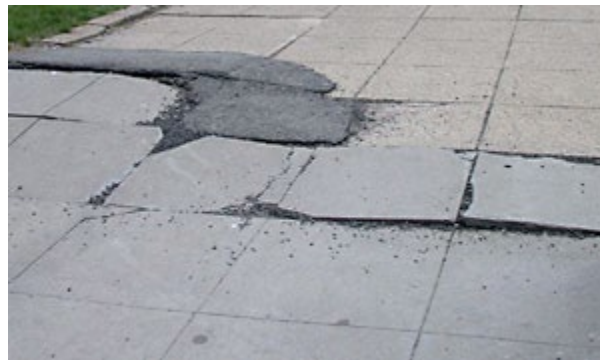
A sidewalk with raised and broken sections is a barrier to access
